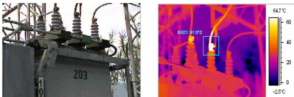
Figure 4. Infrared Thermography of a Recloser
