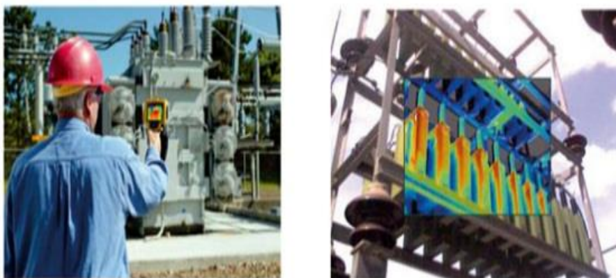
Figure 2. Review of a transformer body and its ventilation systems. Thermography with IR technology Fusion of a capacitor bank.
